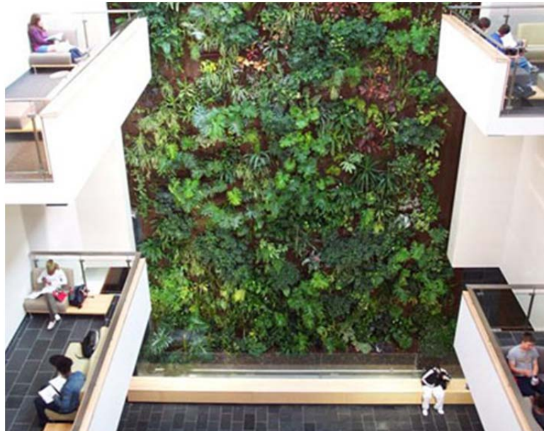
Air Biofilter at University of Guelph, Ontario
