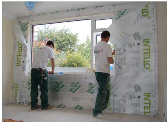
Internal wall insulation being retrofitted correctly with airtightness membrane sealed on the warm side of the insulation to prevent moisture movement to the cold part of the wall.
