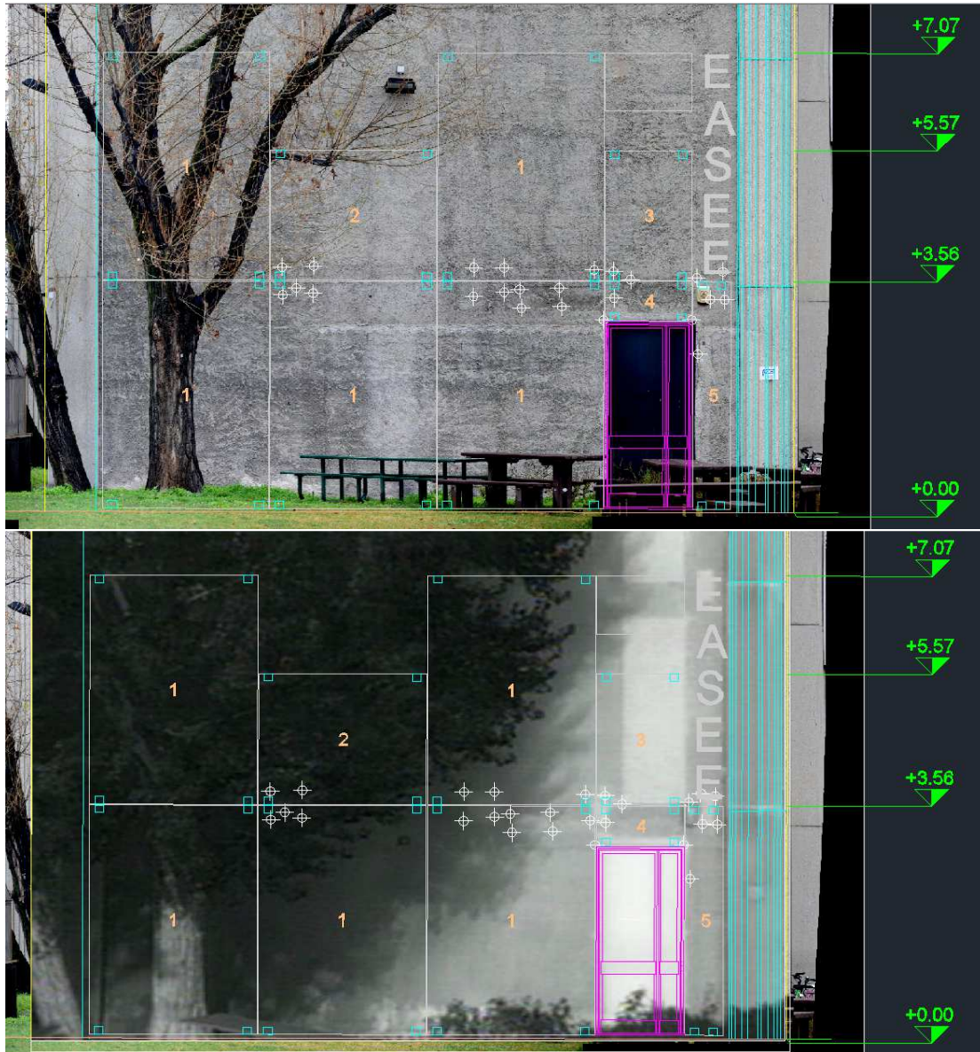
Figure 29: Design of the façade panels overlaid to the thermal orthophoto and the thermal anomalies positioning to support the Design of the panels and the location of the anchors avoiding the whole detected or reinforcing them
