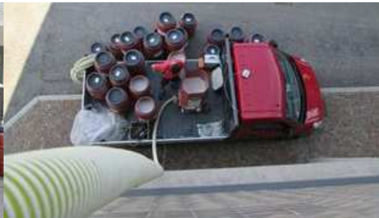
4 - Positioning of the blowing machine on a lorry in order to deliver the loose perlite two floors above.
