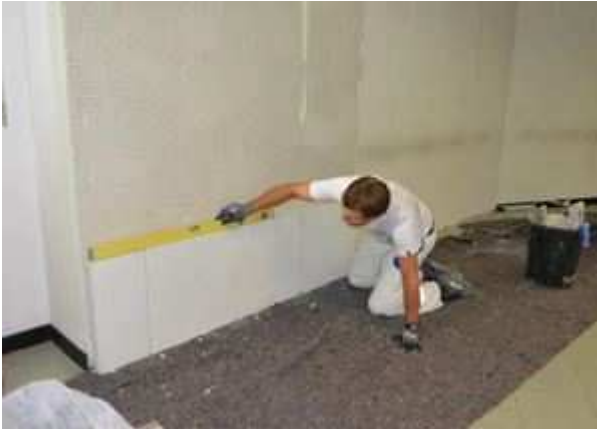
3 - Application of the first line of the perlite insulation boards on the adhesive mortar.
