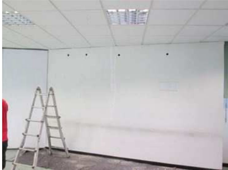
2 - Holes were drilled at the top of the cavity prior the installation of perlite. Because of the latter's granular characteristics, allowing the perlite to seep in the cavity simply by gravity, it was not necessary to drill additional holes at mid-height.
